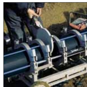
Butt welding is a technique that has been used for several years for mounting PE-pipes
