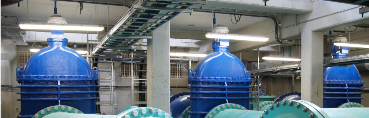
Photograph 3 New AVK DN1200 Series 54 Gate Valves
