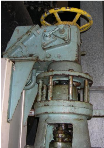
Photograph 6 Original Actuated Valves
