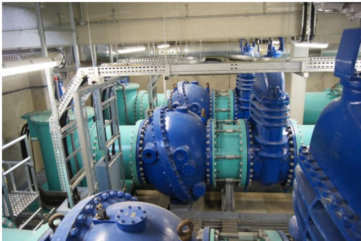
Photograph 4 New AVK Valves Within Pump House
