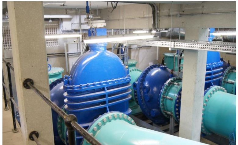
Photograph 5 New AVK Valves Within Pump House
